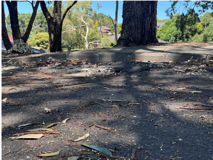
North Terrace roadway and footpath damage
