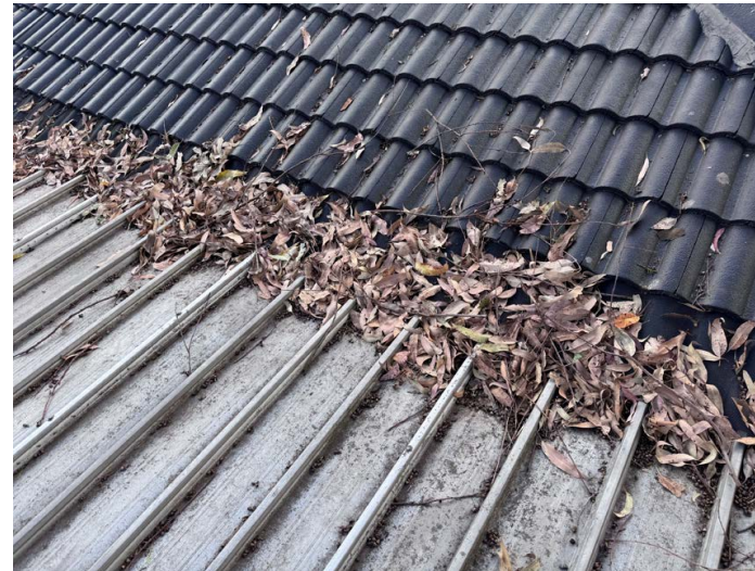
Debris build up on roof
