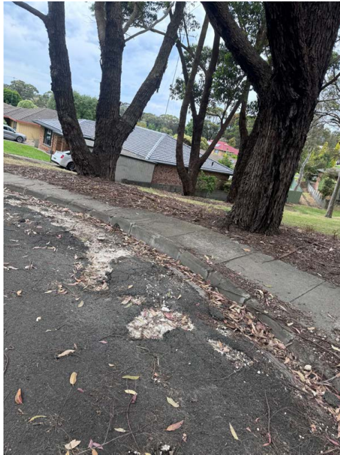
Roadway damaged by tree roots, raised footpath
