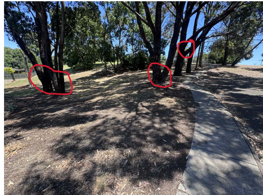
5 trees, dead grass due to trees, multiple cracks showing
