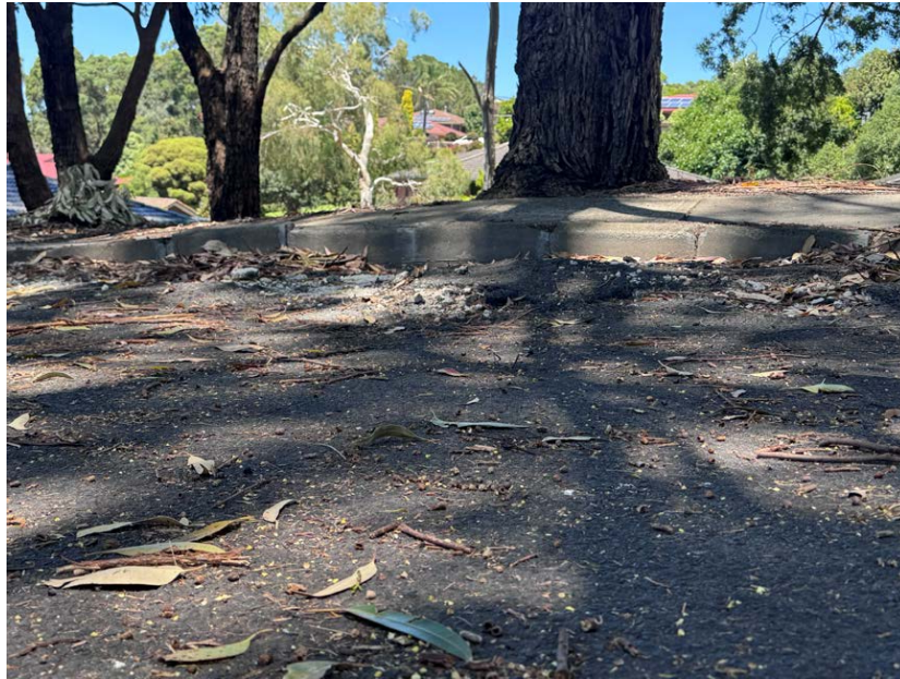
North Terrace roadway and footpath damage
