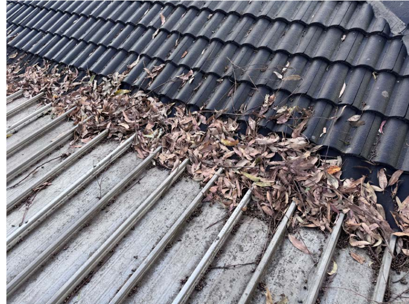
Debris build up on roof
