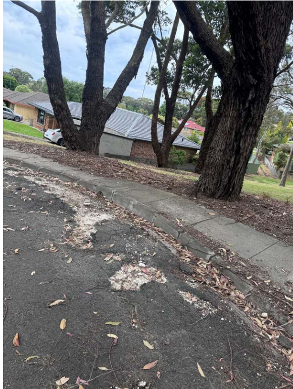
Roadway damaged by tree roots, raised footpath
