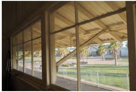
When it is restored, the Signal Cabin will provide 180° views across the Railway Lands
