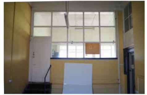
The glazed screen between the Signal Cabin and the Stationmasters Office is not original and should be removed.
