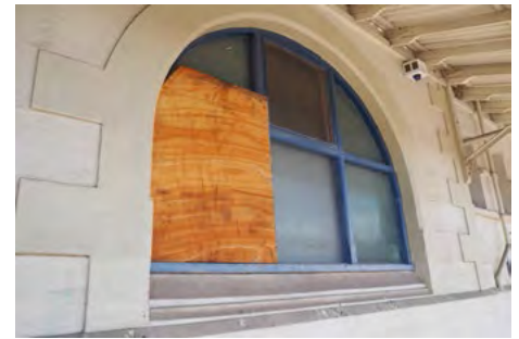
Boarded up and dust windows increase the risks to the building.
