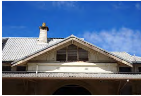
North western gable with metal louvre vents. The asbestos side panels will be replaced.
