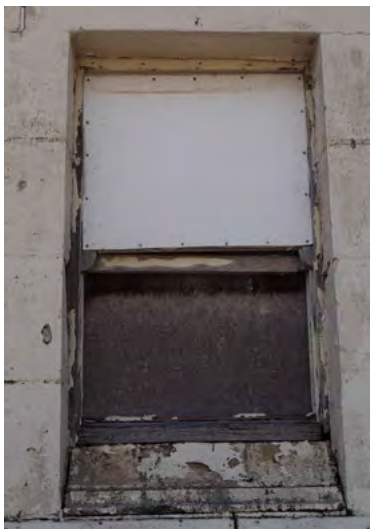
Boarded up toilet window
