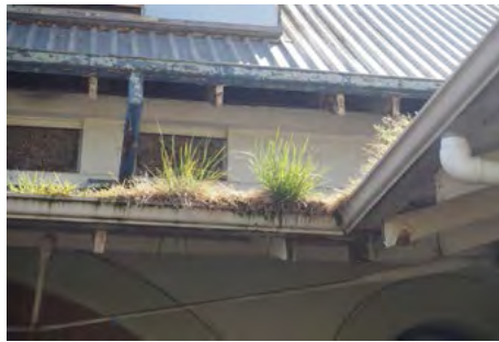
Open bird boards have allowed pigeons to enter. This has led to the gutters being blocked, damaging the structural timberwork.
