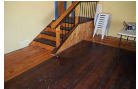
These steps are not original and should be removed. The polished timber floor can remain.
