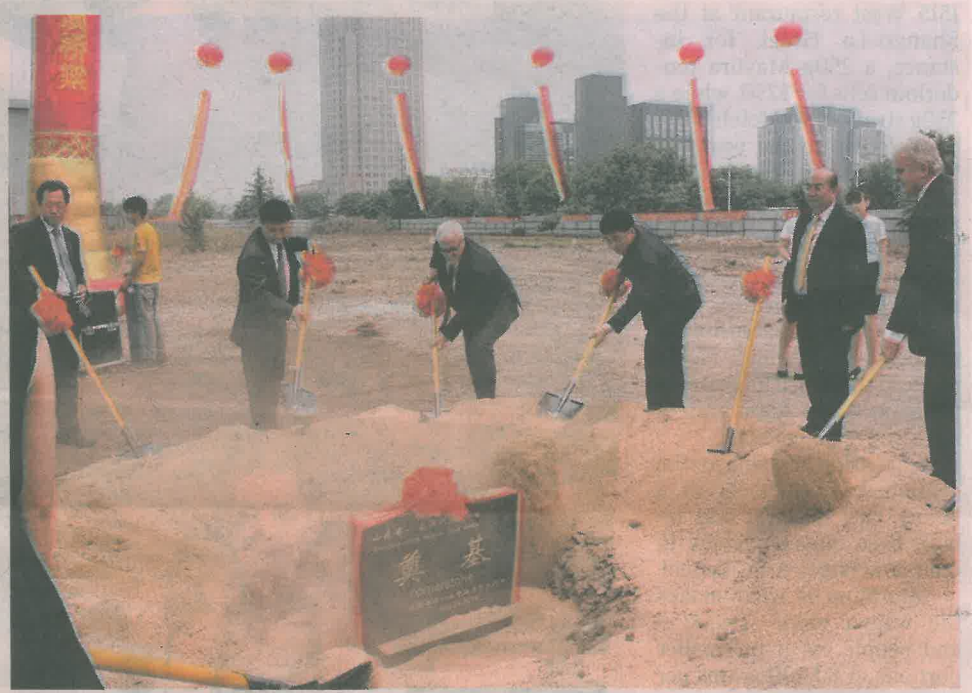
START: Tony Royal, far right, and SA Government representative Rik Morris, centre, help lay the cornerstone of the Shandong-SA International Commerce Centre. Picture: PORTAVIN
